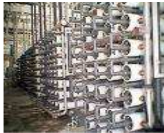
Reverse Osmosis Filtration
